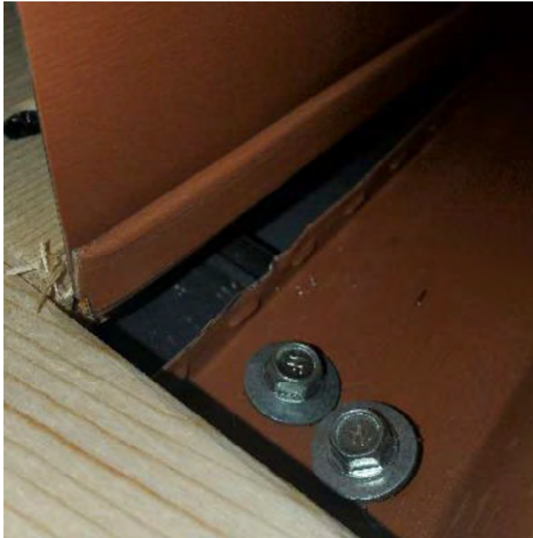
Photo No. 2 Failure Photo #1
