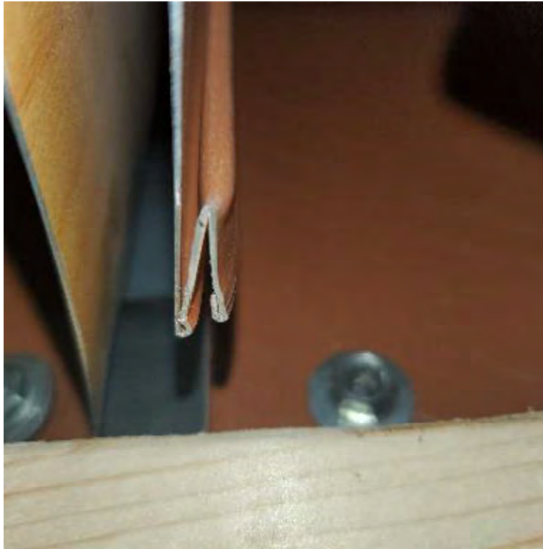
Photo No. 3 Failure Photo #2
