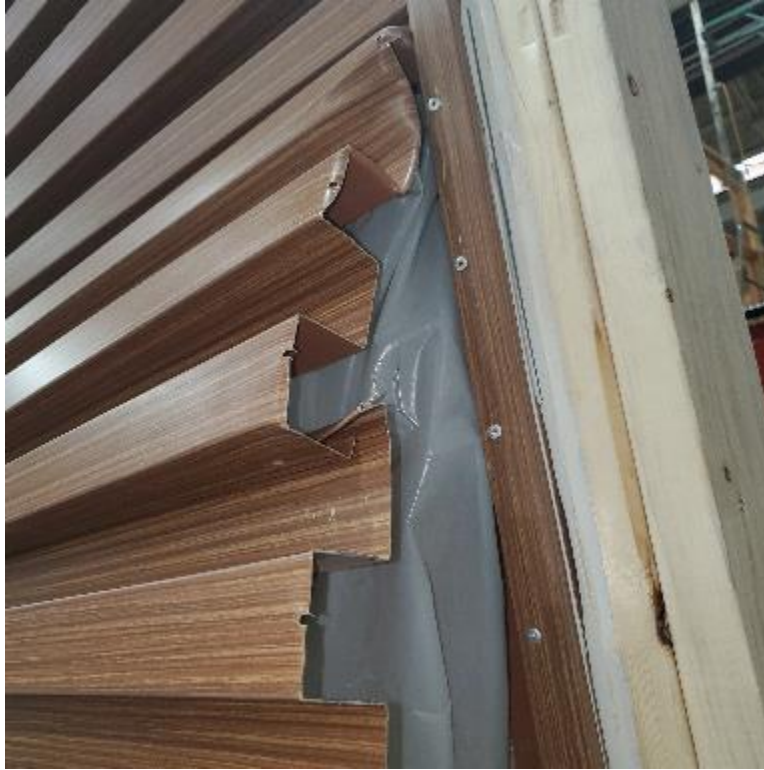
Photo No. 2 Failure Photo #1
